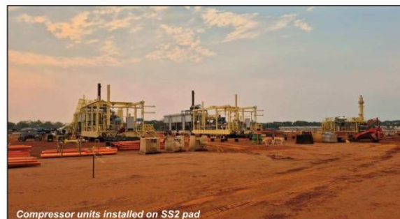
Compressor units installed on SS2 pad
