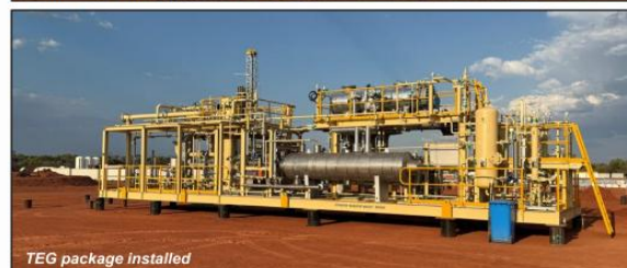
TEG package installed
